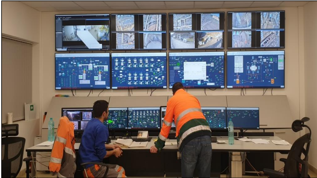
Figure 17-3: Control Room overview Source: DPM, 2020
